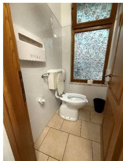
Figure 25 toilet without grab bars
